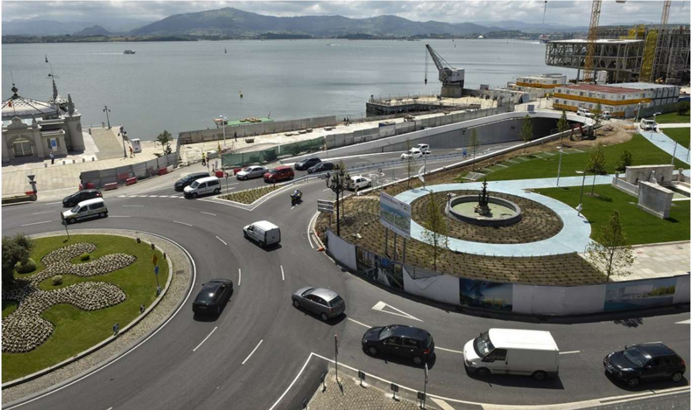
Botín Center building works, example of the transformation of the waterfront. (Photo: City of Santander)
