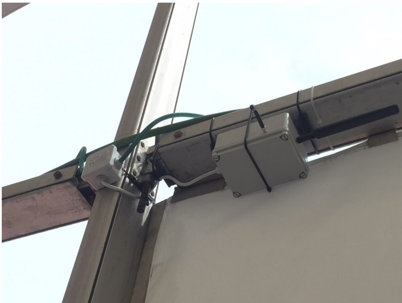
WiFi sensors installed in the cruise terminal. (Source: Fundación Valenciaport, 2021).
