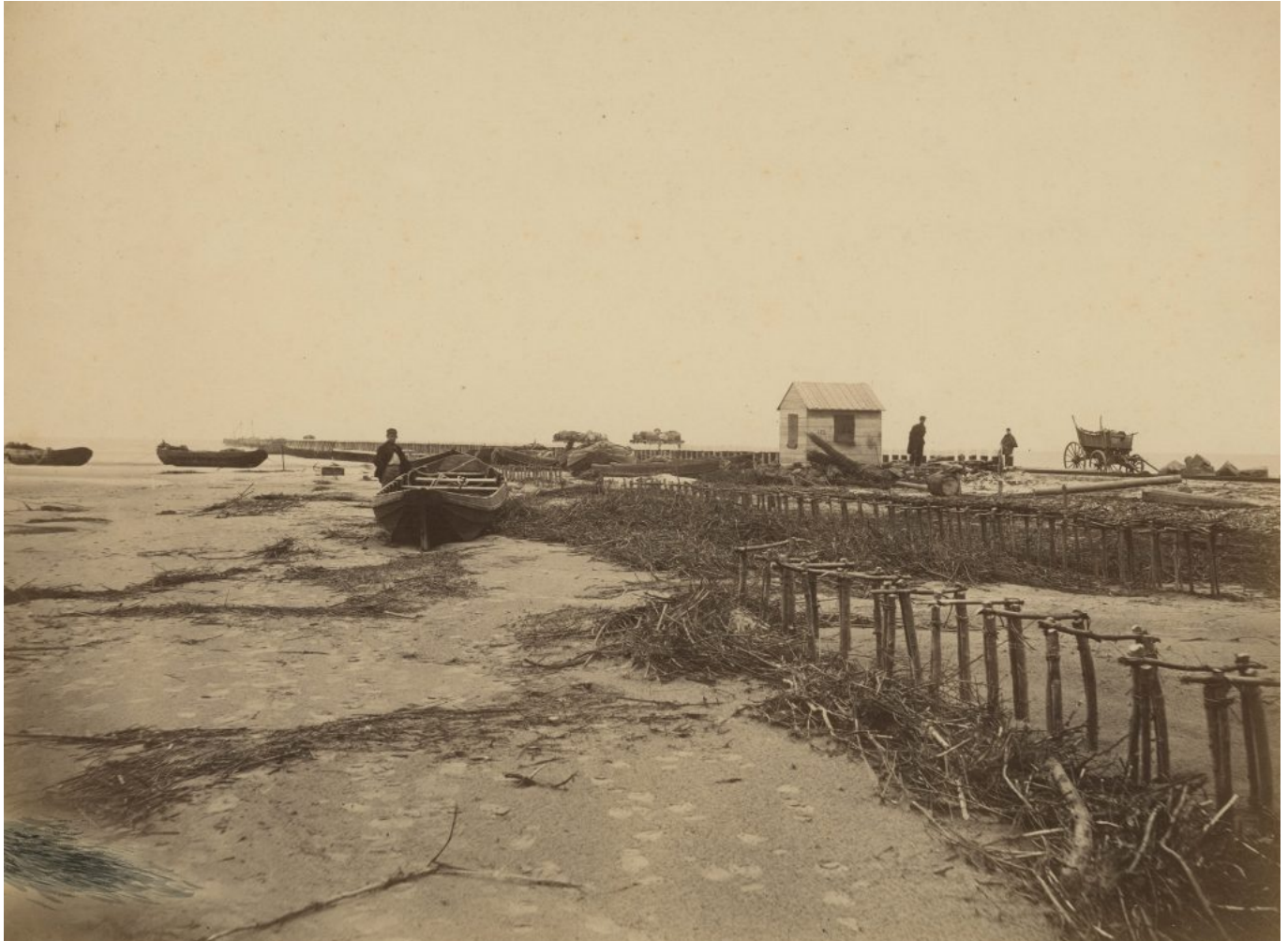
The start of the work on the New Waterway: the construction of the north pier into the sea. (Source: Collection Municipal Archives Rotterdam, number 4187 / XXVIII).
