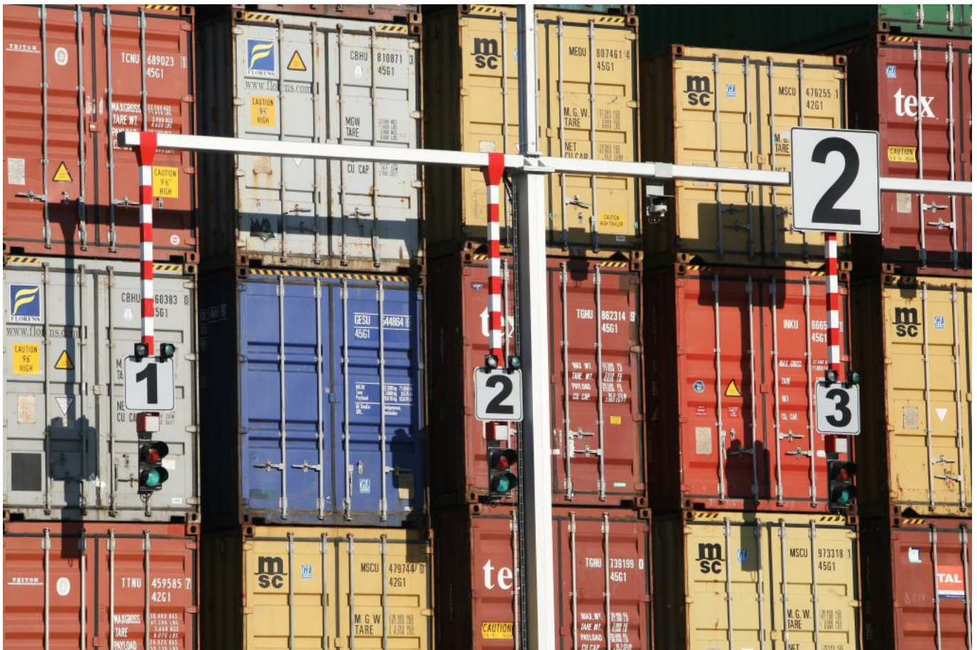
Devices for presence detection and traffic regulation in the maritime transfer area of the ASC blocks. (© Barcelona Europe South Terminal - BEST).
